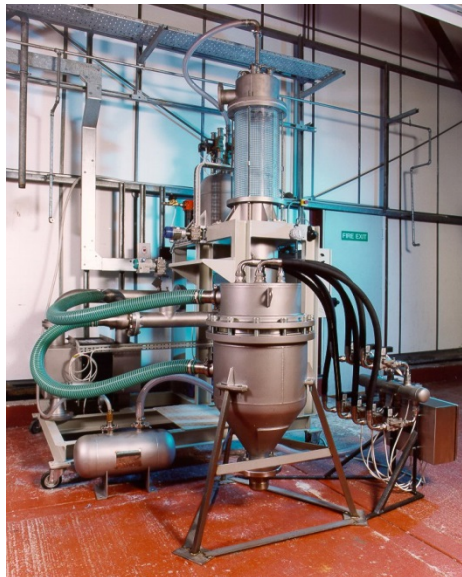
Fig. 5 MOX Pellet Grinding PulseJet Filter installed in test and development Facility
