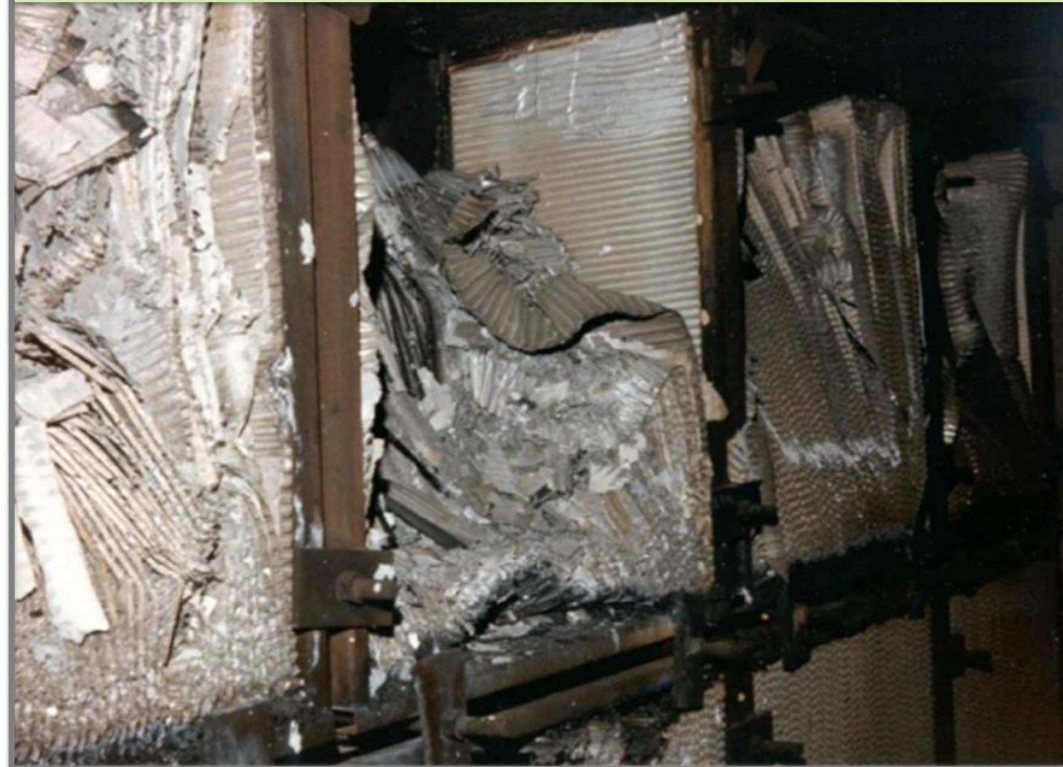
Water damage to filters following a fire
