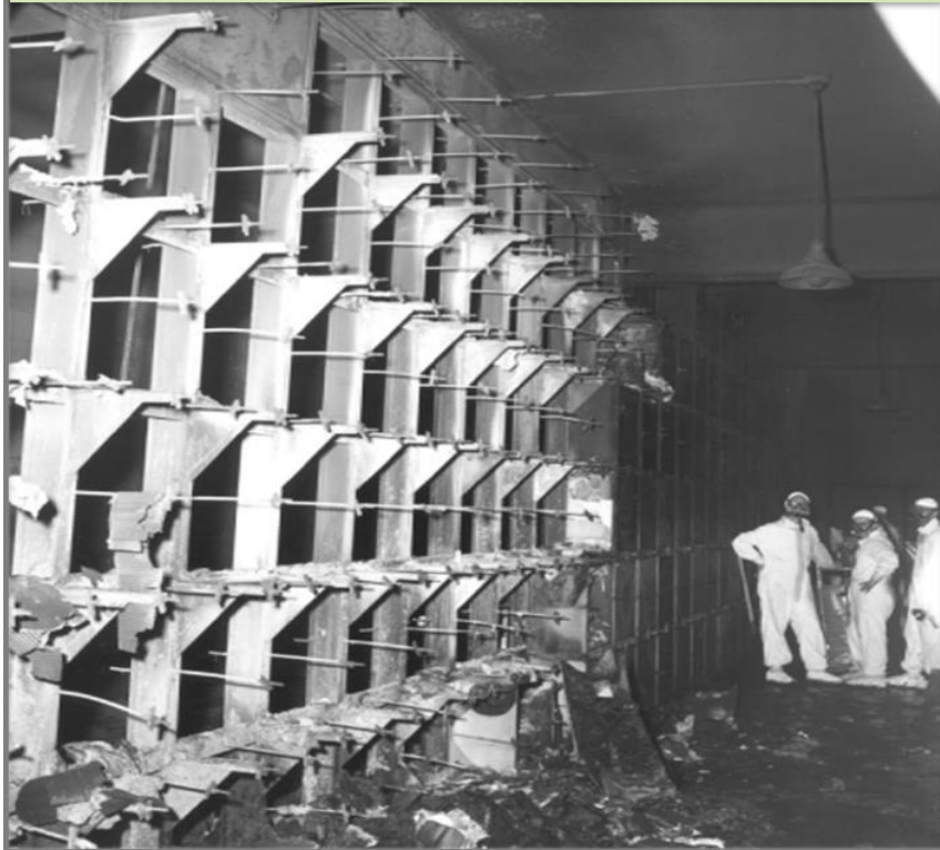
Destroyed filter bank after a fire
